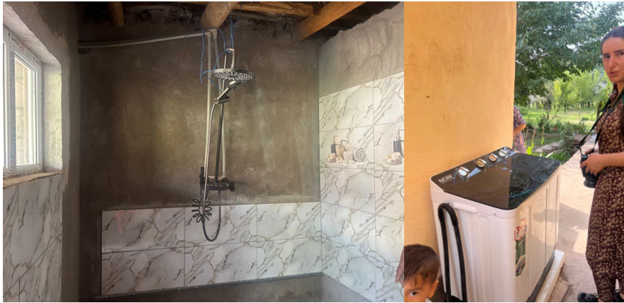
Figure 12: Additional infrastructure installed connected to solar water heaters
