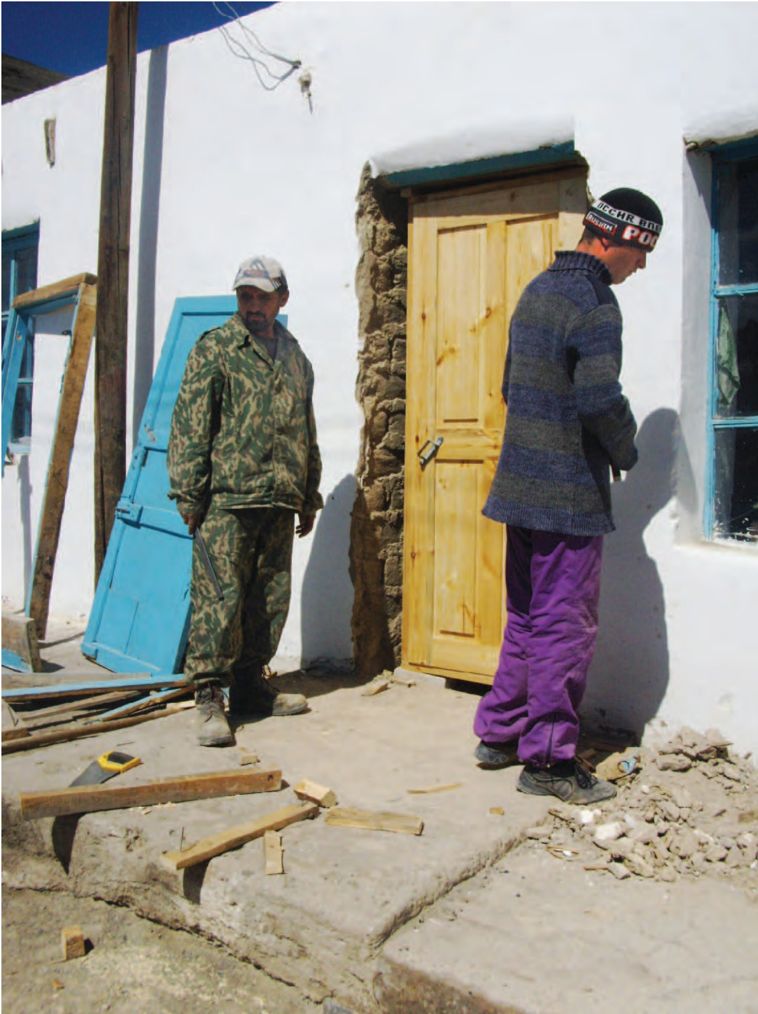
FIGURE 3 Construction workers in Murgab are installing a hermetically closing wooden door produced by carpenters in Khorog. (Photo by Rustam Zevarshoev 2010)
