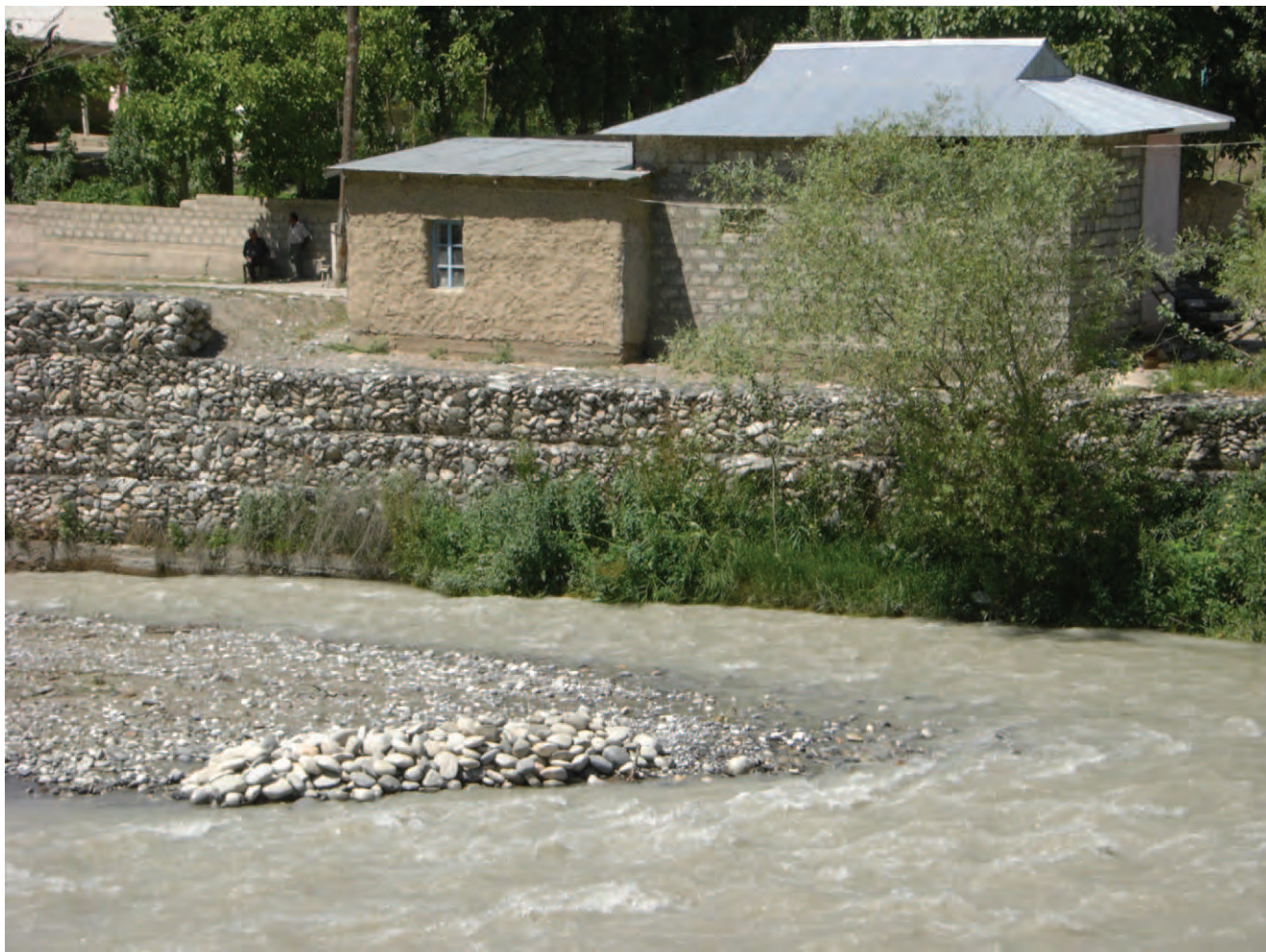
FIGURE 7 In the upper part of the watershed, stonewalls have been constructed to protect homes close to the riverbank from flash floods. Khozho-Bakyrghan WUA, Kyrgyzstan. (Photo by Dominic Stucker, 2011)
