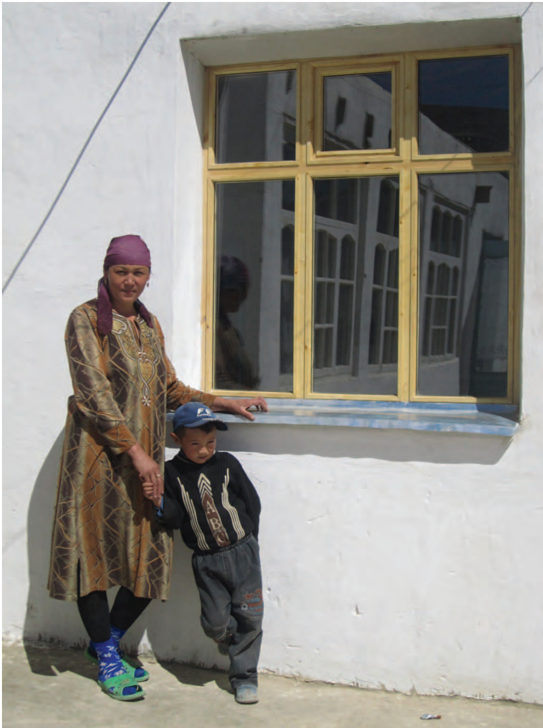
FIGURE 4 The new wooden windows are double glazed and hermetic. In the past, many windows were only single glazed, had broken glass, and were covered with plastic foil during winter to reduce the loss of heat. (Photo by Stefan Salzmann, 2010)
