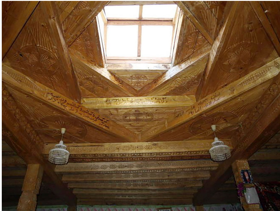
Photo 3 and 4. Ceiling construction of a Pamirian house: the first photo – antique building with swastikas carved during Navruz (from the author's archive).
